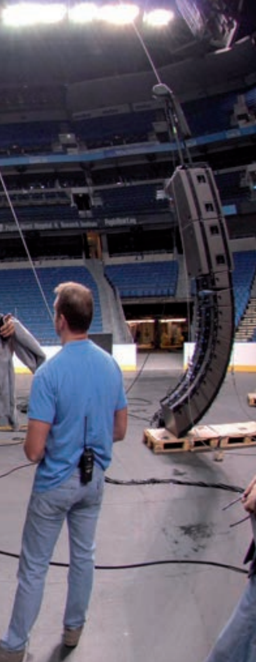
▲ The installation of the sound system at Amalie Arena could be completed in three days to meet busy sports facility calendars, with amazing results.
